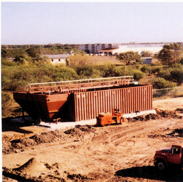
Smith & Loveless' field subcontractors erect this Field-Erected ADDIGEST quickly. Its bolt and weld together design keeps erection and installation time at a minimum.
